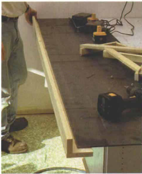
Concrete covers the edge of the steel. By pulling the edge of the form 1 in. away from the steel, Story ensures that concrete will hide the rough edge.
