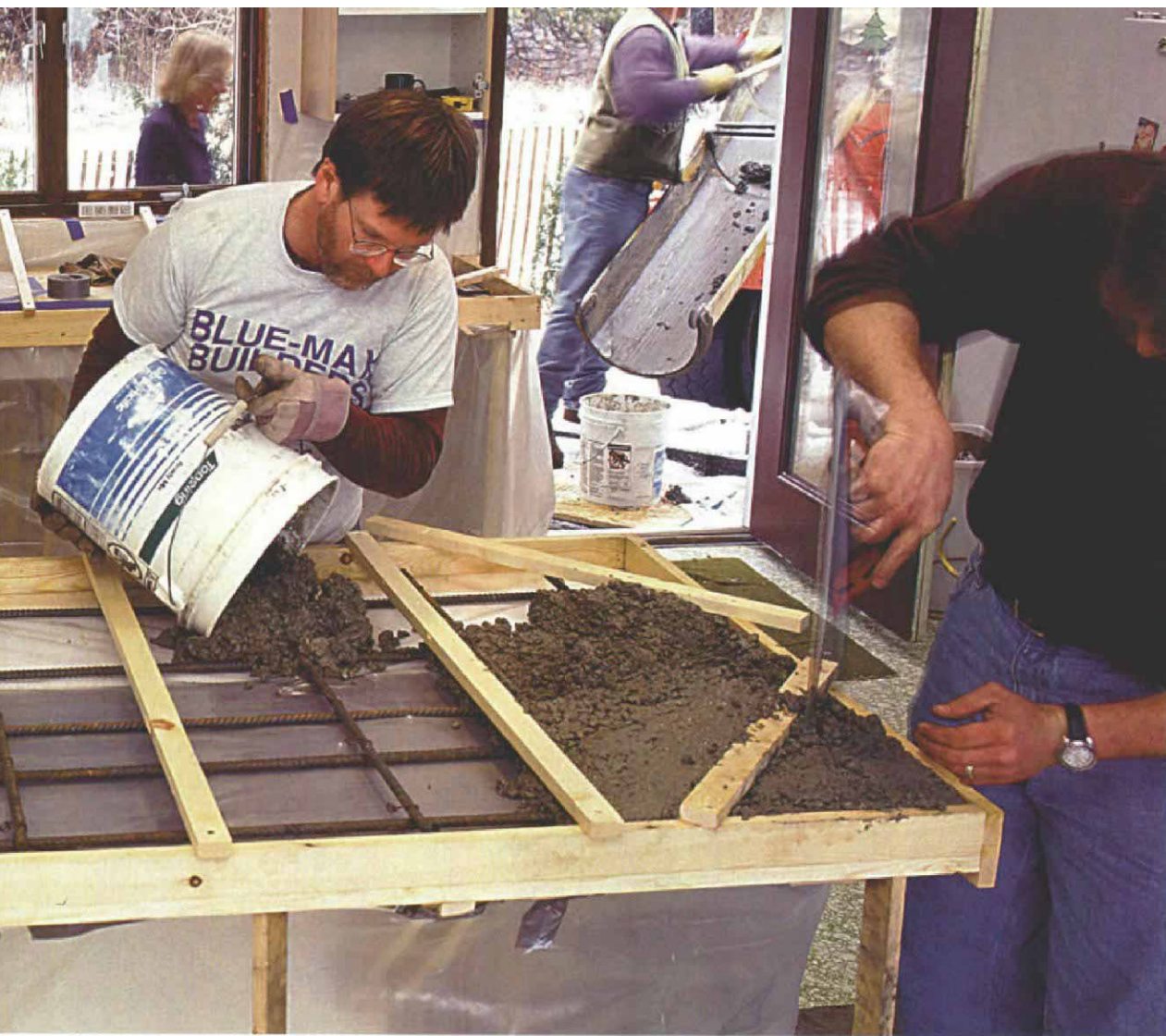
The right mix for a countertop. The author dumps ready-mix concrete into forms built over a set of frameless kitchen cabinets. When cured and finished with an acid-based stain (inset photo), the counter looks like burnished leather.
